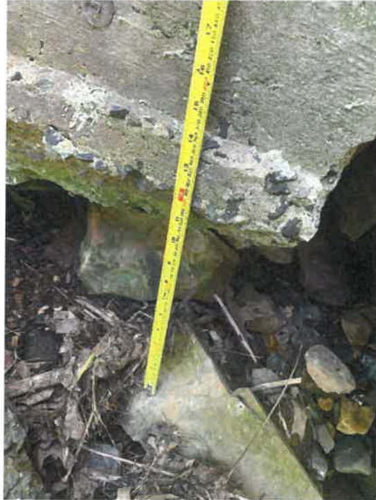
Figure 6 – Erosion at Culvert Wall
