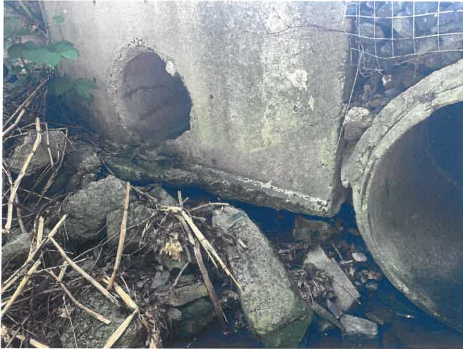
Figure 7 – Broken Concrete Floor
